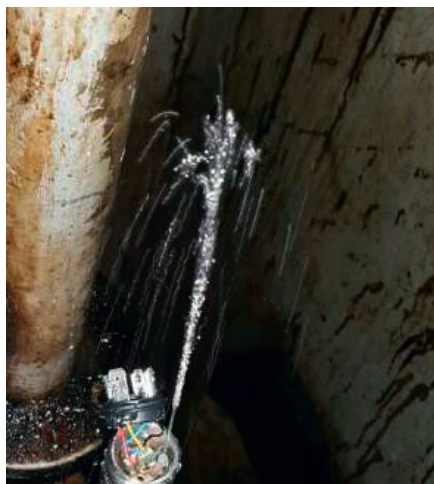
Leakage due to damaged sensor membrane in a water pump.
